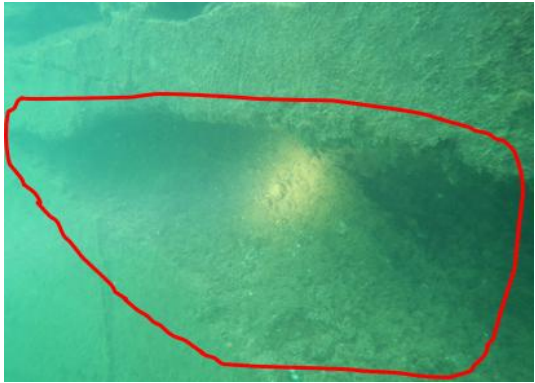
1#墩承台巴马面破损
