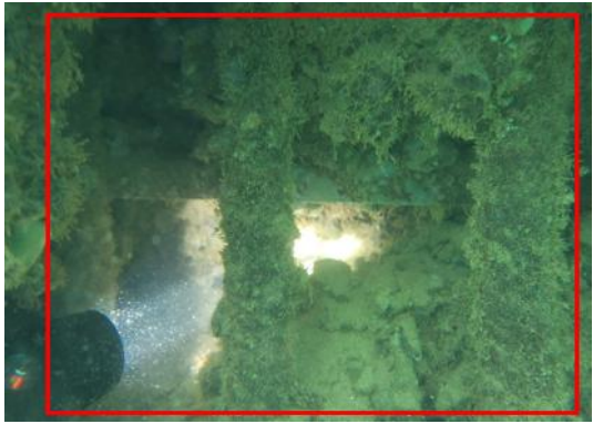
1#墩承台福州面与右侧面斜面处破损、露筋
