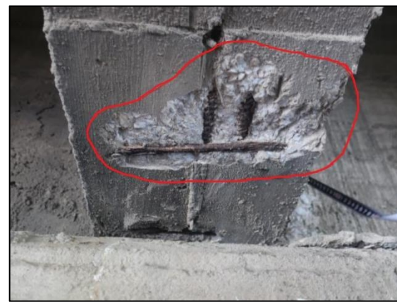
剥落、露筋且锈蚀
