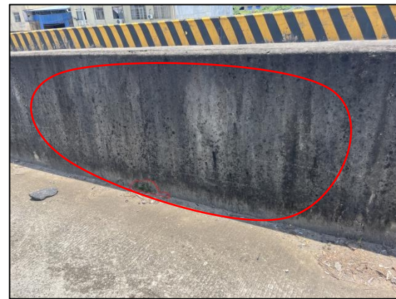
护栏剥落、露筋锈蚀
